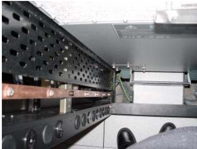
Figure 3. Detail for rear right of Rack A More detail
